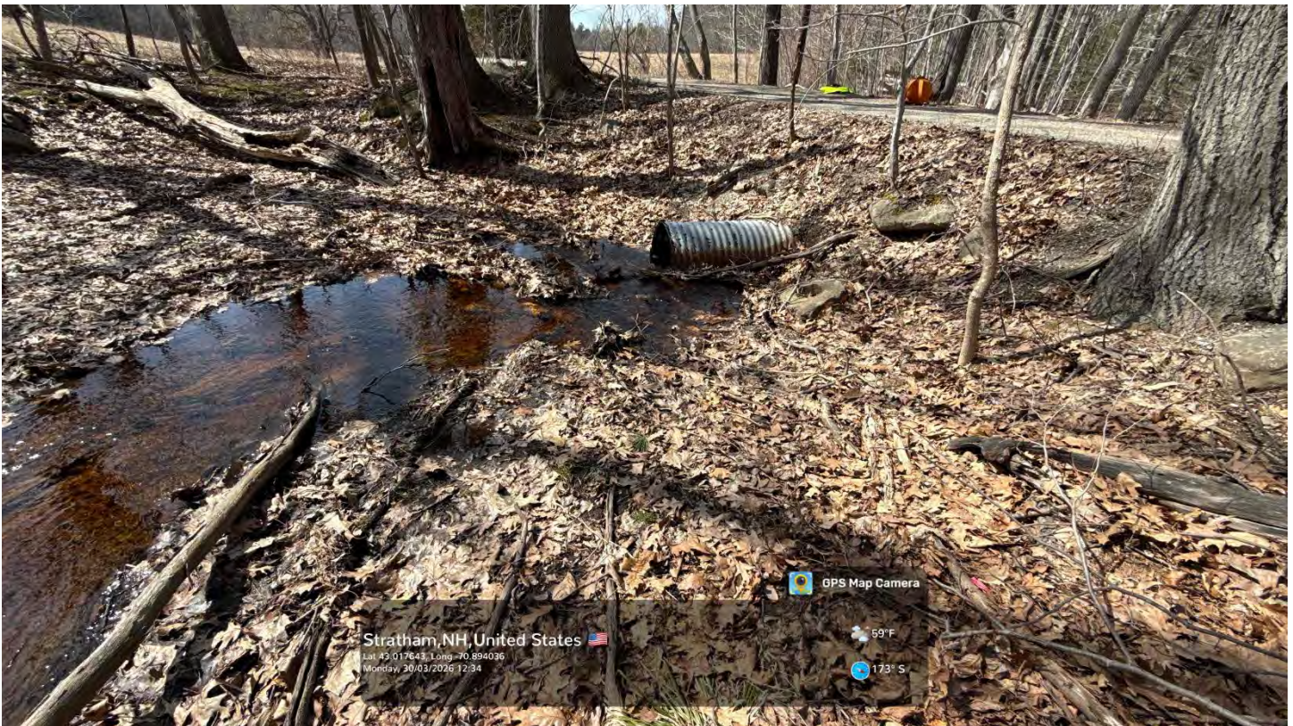
Photo #4: Looking south at same impact area.
