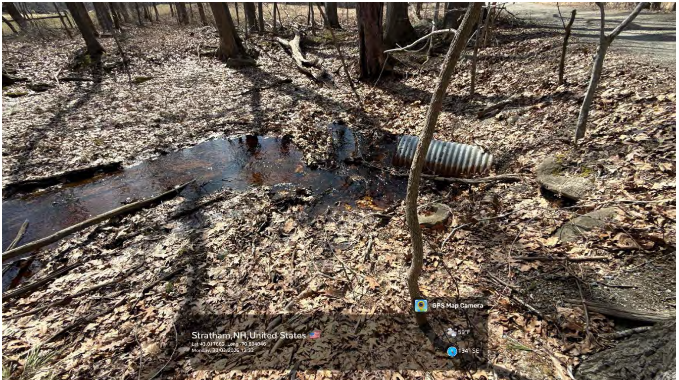
Photo #2: Looking east at same impact area.
